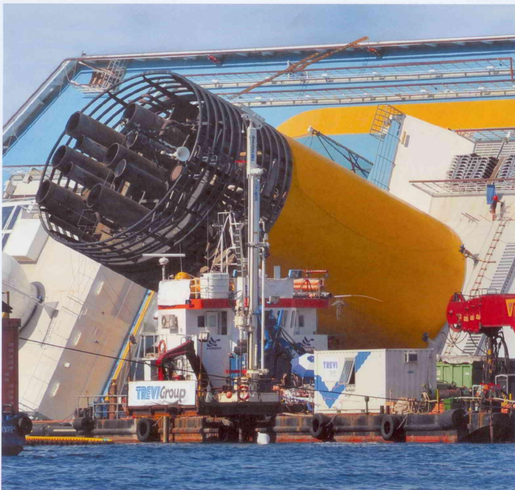
RCT worked off a barge-mounted Soilmec SM-20 drilling rig placed along side the ship's hull.
