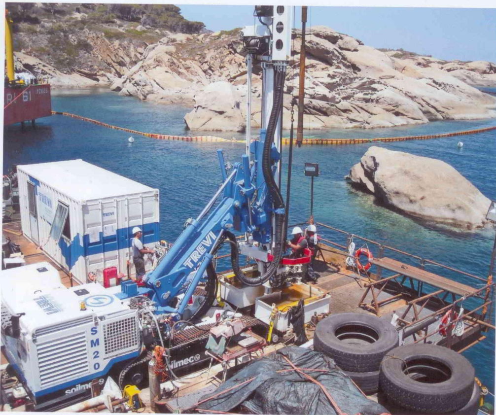
A Soilmec SM-20 microdrilling rig was used for the subsurface investigation into granitic rock.
