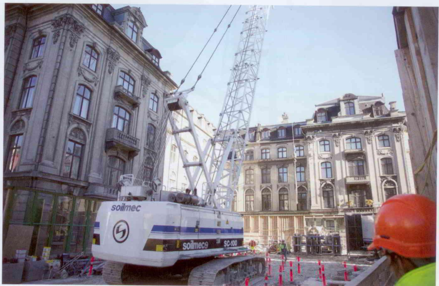
Trevi workers construct cased auger piles near the Marmorkirken (Marble Church). Monitoring with Soilmecc's Drilling Mate System helped ensure that this historic church was left undisturbed.
