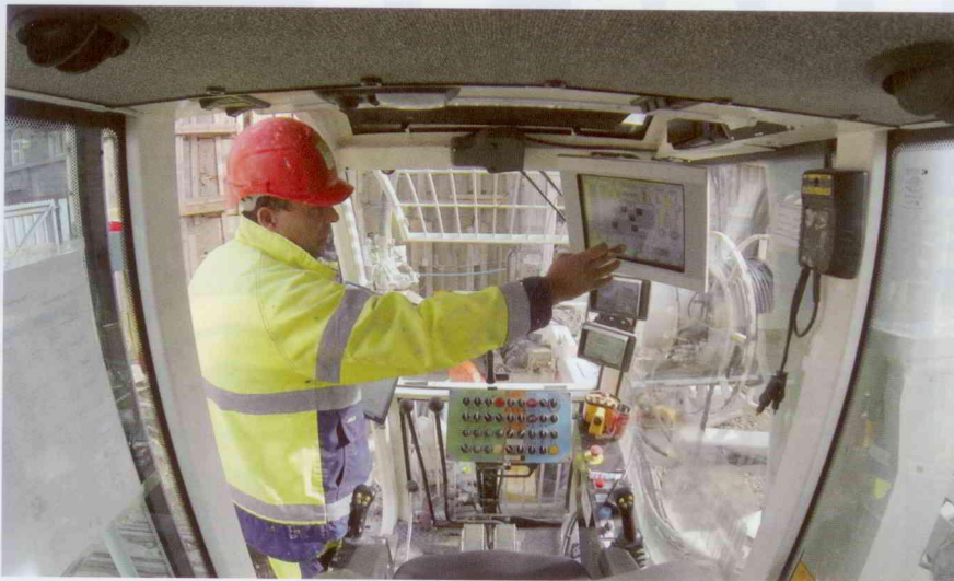
A Trevi worker uses Soilmecc's Drilling Mate System to monitor the hydromill diaphragm wall construction in Copenhagen.
