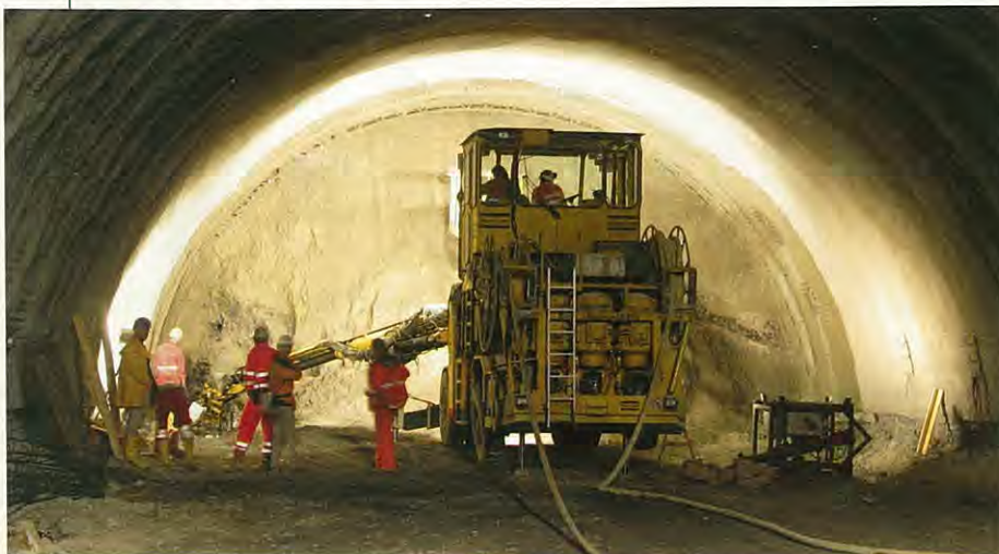
Left: Drill and blast on the longer tunnel section from Stans to Terfens village
