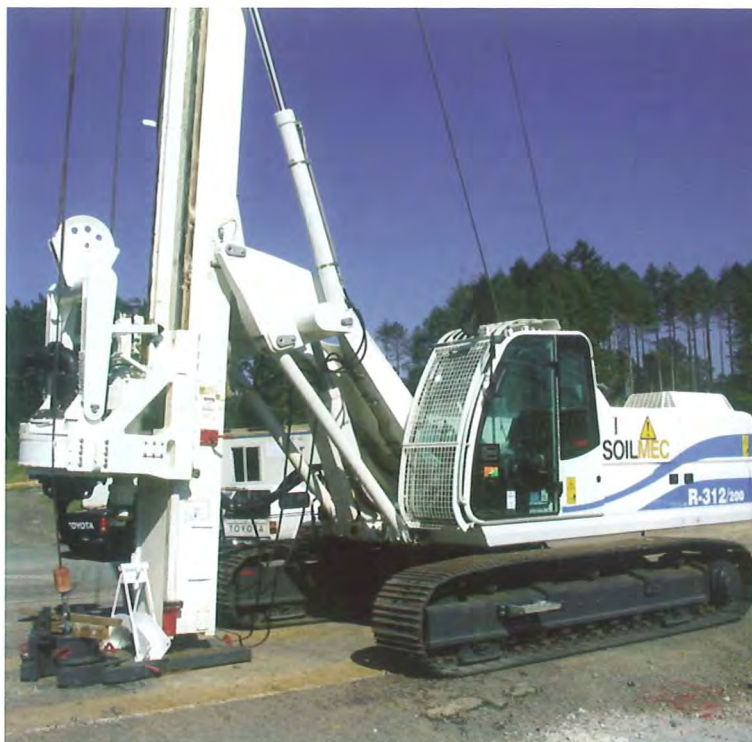
LEFT: Various Trevi and Brian Perry Civil machines at work on the dam crest.
