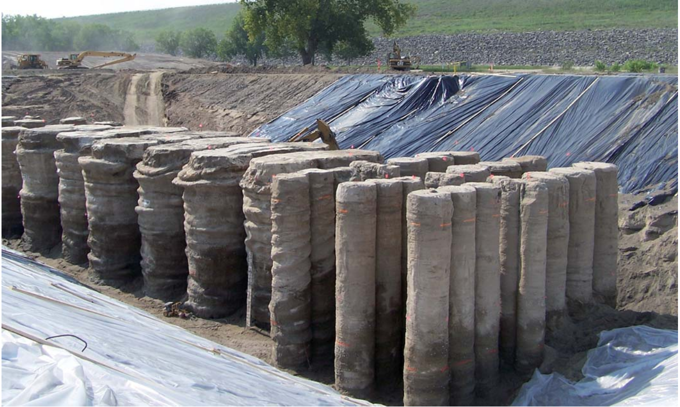
Test field at Tuttle Creek Dam (KS, USA). The geometry of triple fluid jet grouting columns installed (on the left hand side) reflect the consistency of the soil, whereas the DMM columns (right hand side) have a perfectly cylindrical shape.
